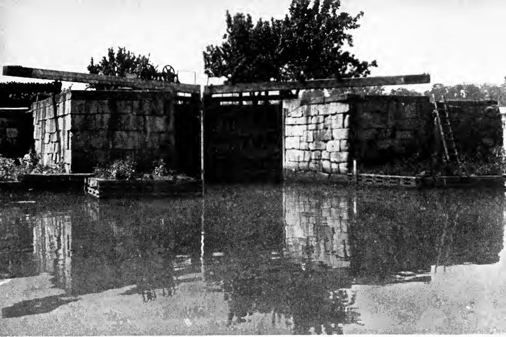
Old Schuylkill Navigation Canal Lock in Fairmount Park "Along its path the straining tow mules plodded"
